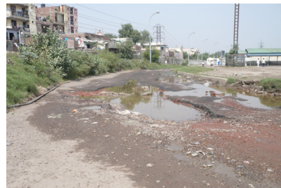
Poor drainage condition
